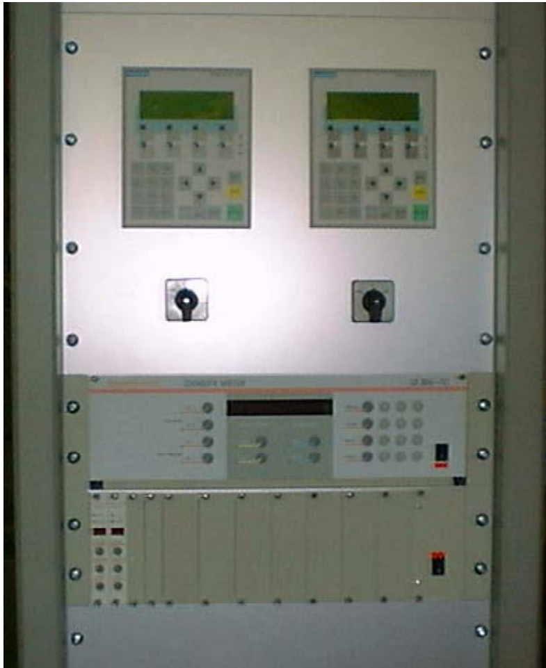
Cabinet with Evaluation Unit and Motor Controls
